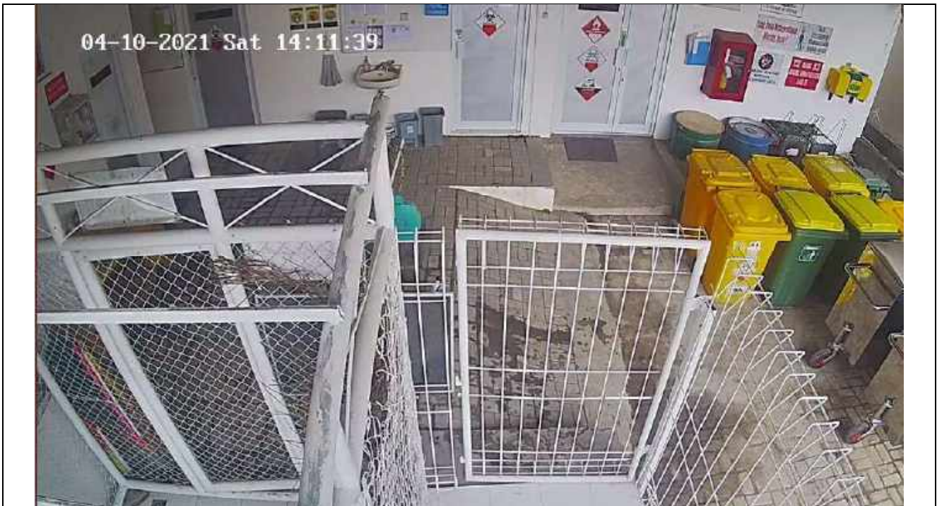
Figure 3. The temporary waste storage for hazardous wastes (Asr Medical Center Hospital, Universitas Muhammadiyah Yogyakarta, Indonesia)
