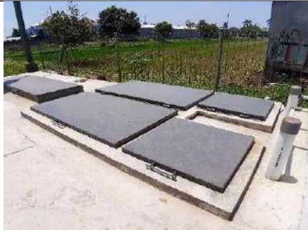
Figure 2. Underground water tanks for recycled water in Universitas Muhammadiyah Yogyakarta
