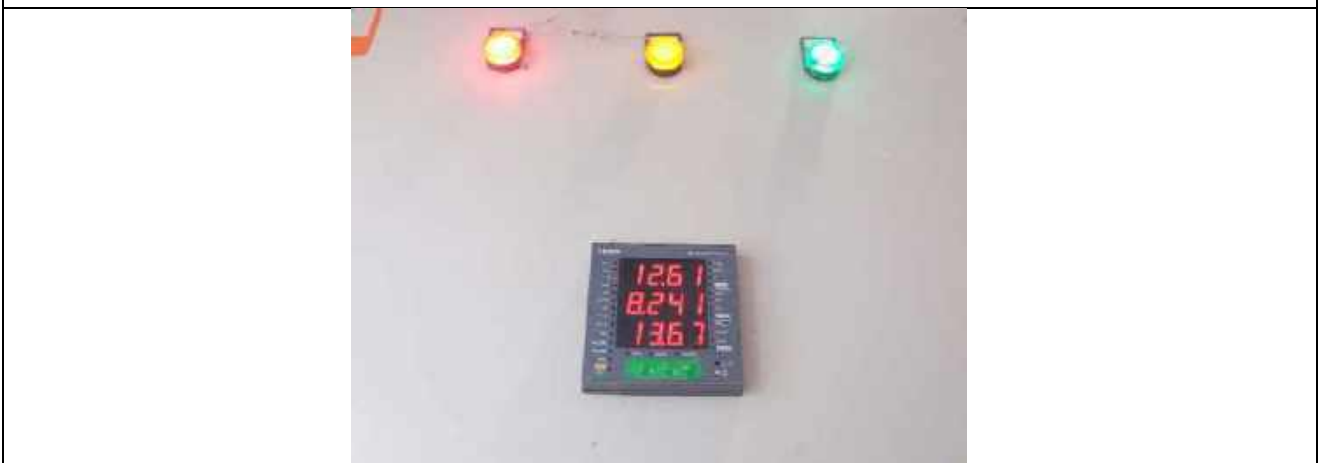
Figure 6. Submetering in Universitas Muhammadiyah Yogyakarta Buildings (Admission Building)
