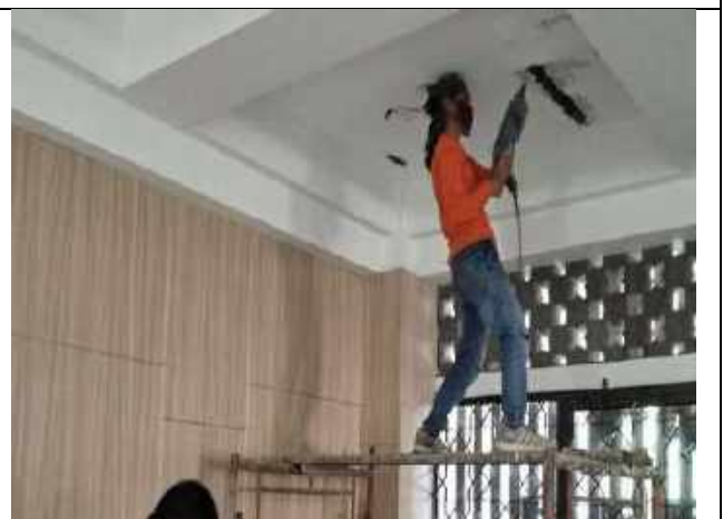
Figure 6. Operation of Ceiling
