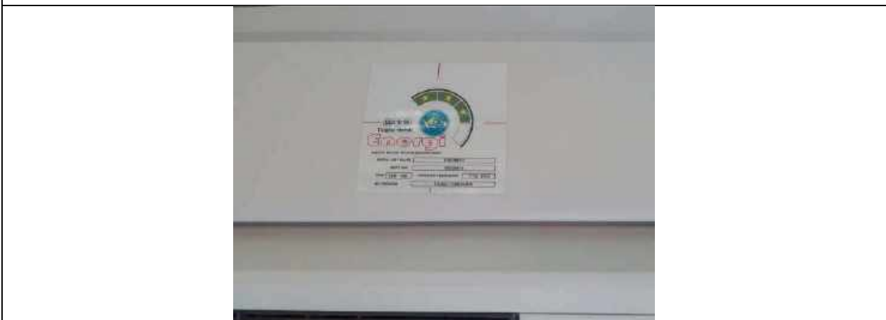
Figure 5. Air conditioning with the energy-efficient label
