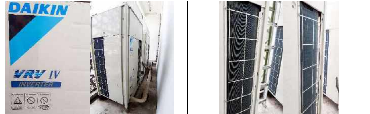
Figure 4. Air conditioning with VRV technology
