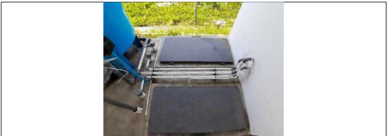
Figure 1. Water tank for wastewater collection
